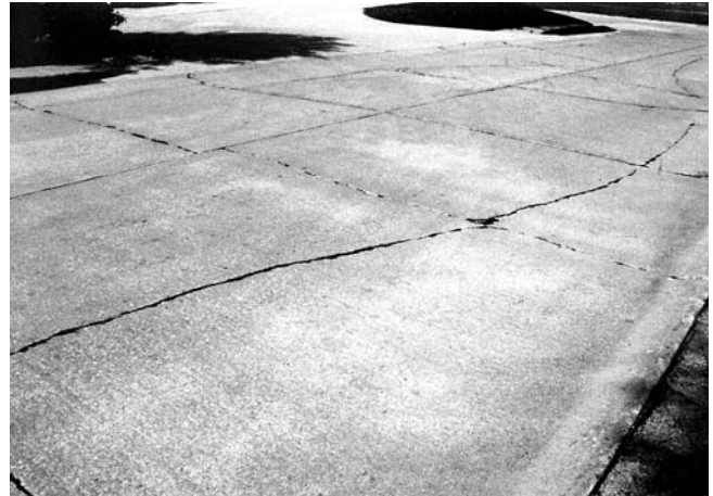
FIG. X2.7 Low-Severity Divided Slab
