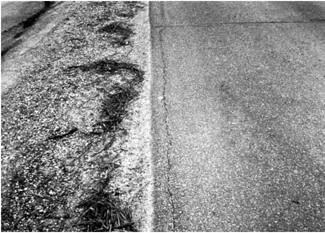
FIG. X1.19 Low-Severity Edge Cracking
