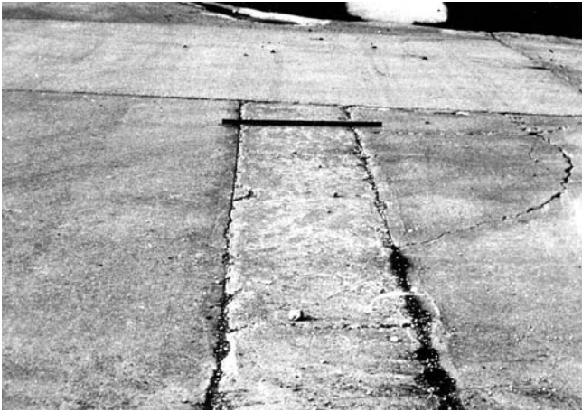
FIG. X2.26 Medium-Severity Patching, Large and Utility Cuts
