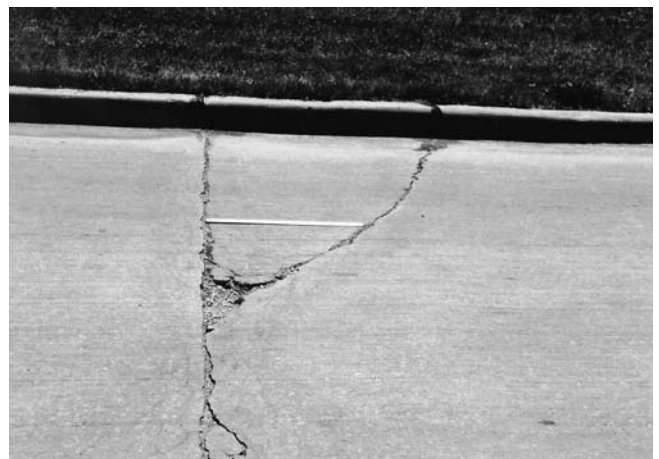
FIG. X2.5 Medium-Severity Corner Break
