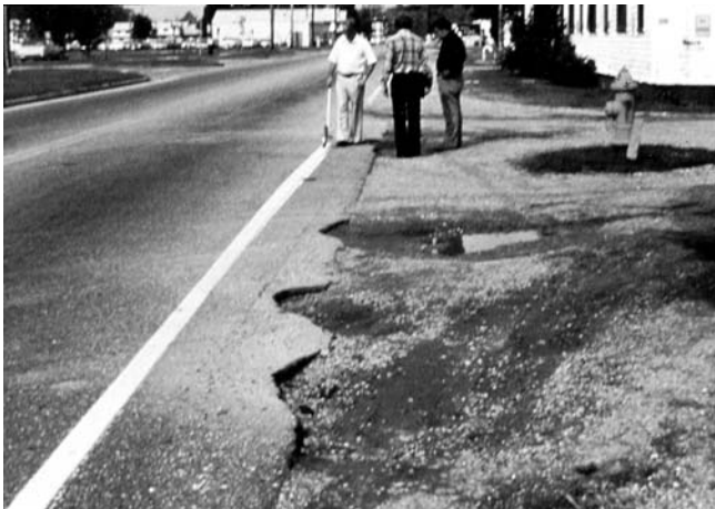
FIG. X1.21 High-Severity Edge Cracking
