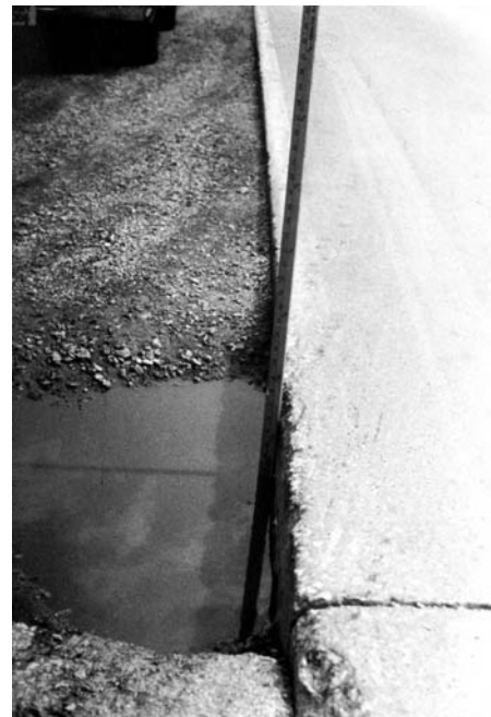
FIG. X2.21 High-Severity Lane/Shoulder Drop-Off
