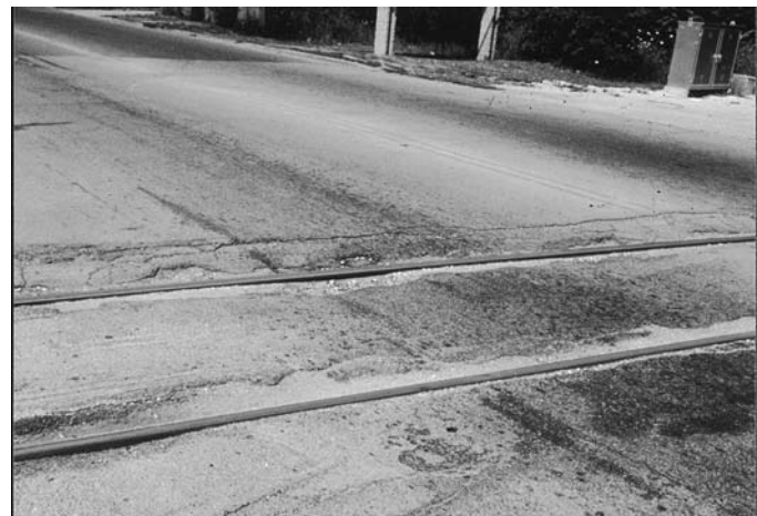
FIG. X1.39 Medium-Severity Railroad Crossing
