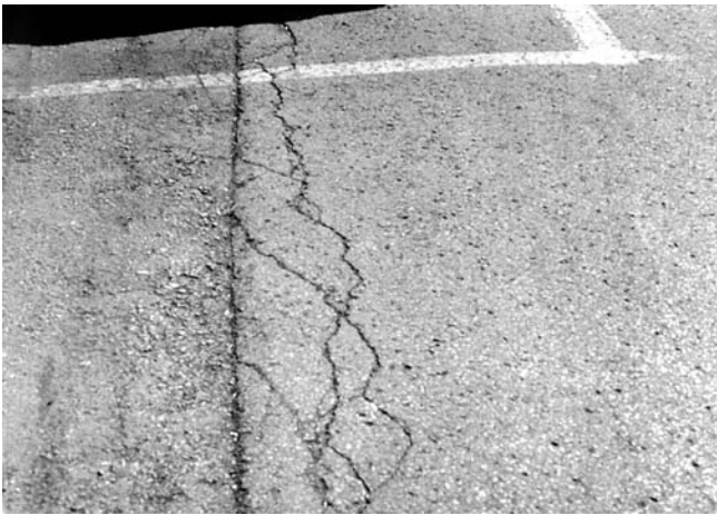
FIG. X1.20 Medium-Severity Edge Cracking
