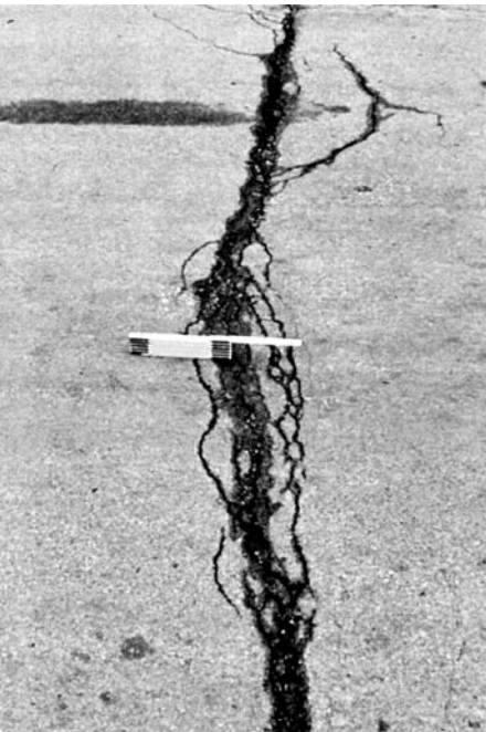
FIG. X1.24 High-Severity Joint Reflection Cracking
