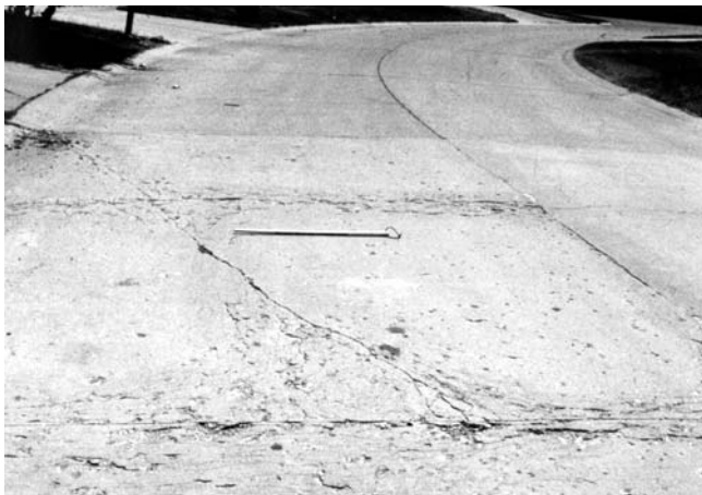
FIG. X2.12 High-Severity Durability Cracking
