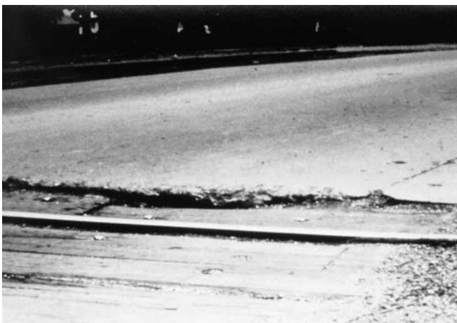
FIG. X2.40 High-Severity Railroad Crossing
