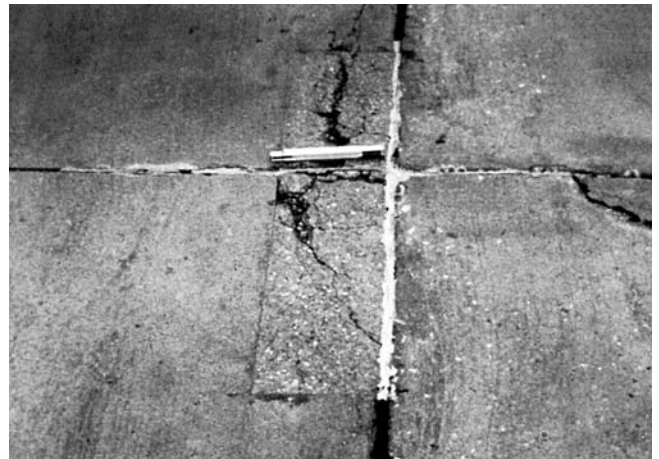
FIG. X2.30 High-Severity Patching, Small
