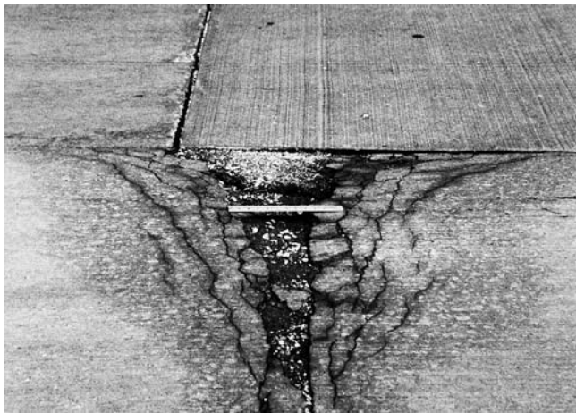
FIG. X2.11 Medium-Severity Durability Cracking
