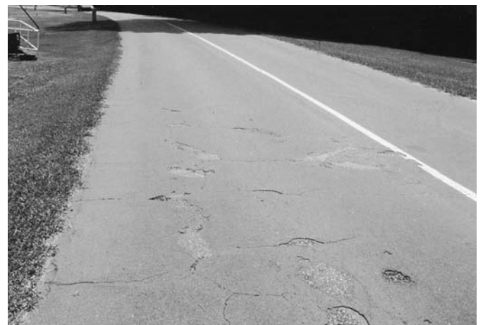
FIG. X1.53 High-Severity Weathering and Raveling
