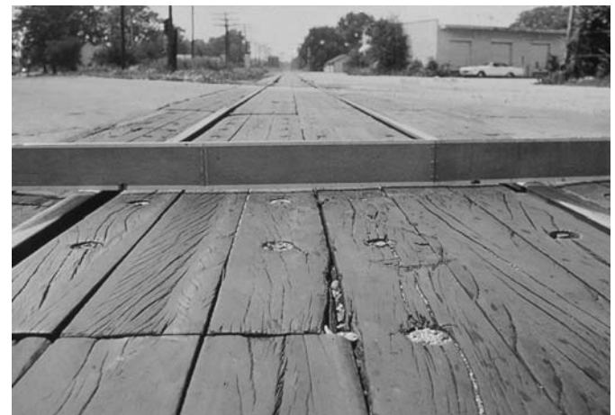
FIG. X1.38 Low-Severity Railroad Crossing
