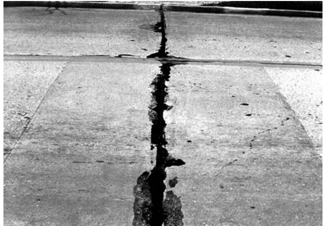
FIG. X2.16 Low-Severity Joint Seal Damage
