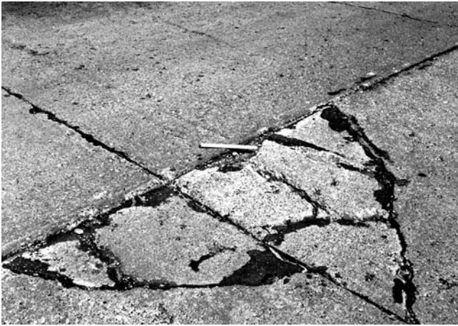
FIG. X2.6 High-Severity Corner Break
