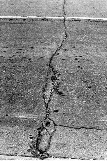
FIG. X1.23 Medium-Severity Joint Reflection Cracking
