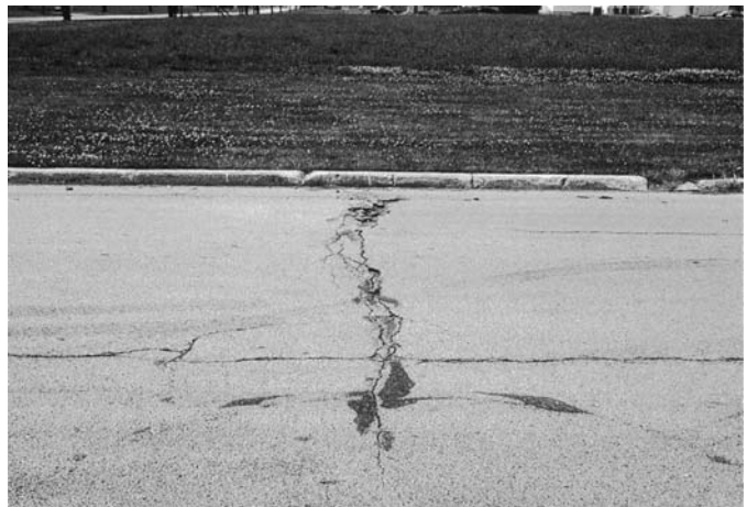
FIG. X1.30 High-Severity Longitudinal and Transverse Cracking
