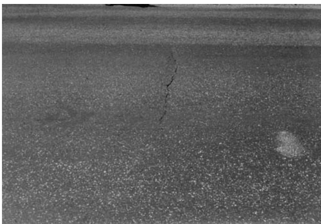
FIG. X1.28 Low-Severity Longitudinal and Transverse Cracking
