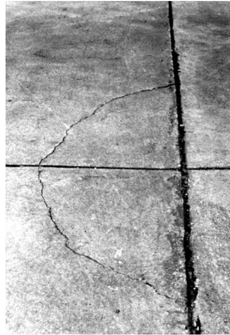
FIG. X2.4 Low-Severity Corner Break
