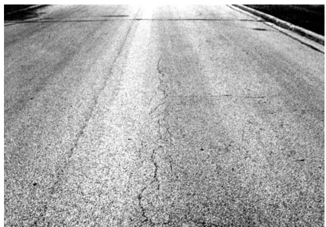
FIG. X1.1 Low-Severity Alligator Cracking
