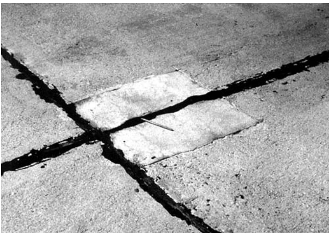
FIG. X2.28 Low-Severity Patching, Small
