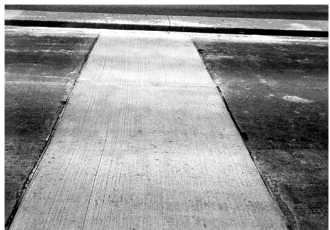
FIG. X2.25 Low-Severity Patching, Large and Utility Cuts
