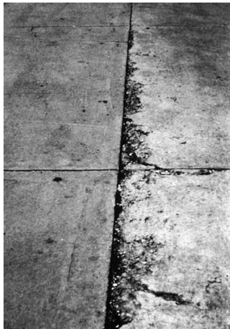
FIG. X2.49 Medium-Severity Spalling, Joint
