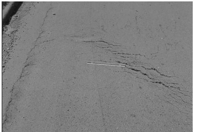
FIG. X1.48 Medium-Severity Slippage Cracking
