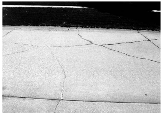
FIG. X2.8 Medium-Severity Divided Slab
