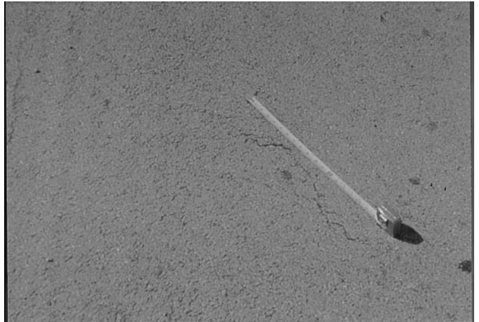
FIG. X1.47 Low-Severity Slippage Cracking
