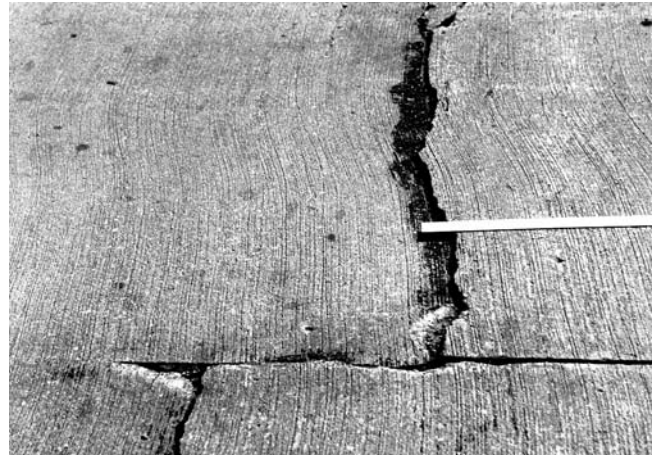
FIG. X2.24 High-Severity Linear Cracking
