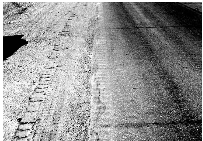
FIG. X1.22 Low-Severity Joint Reflection Cracking
