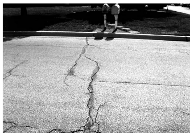
FIG. X1.8 Medium-Severity Block Cracking
