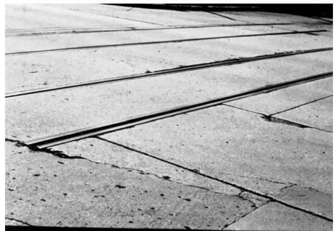
FIG. X2.38 Low-Severity Railroad Crossing
