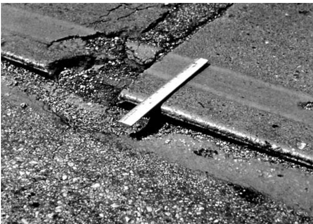
FIG. X2.19 Low-Severity Lane/Shoulder Drop-Off
