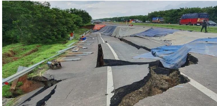
Gambar 1. Lokasi Longsor Jalan Tol Cipali KM122
