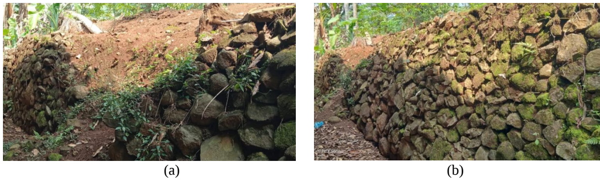
Gambar 1 . Lereng Eksisting: (a) Gerusan Lereng; (b) Eksisting Dinding Penahan
