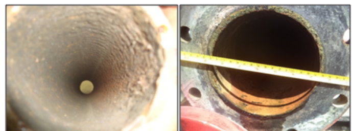
Figure 1. Internal Pipe Condition 3" and 6"
