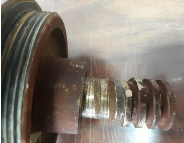
Figure 2. Stem valve that experience a fracture condition
