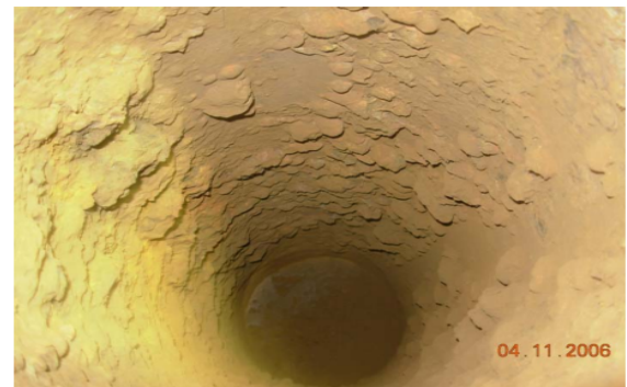
Figure 13. Internal surface condition of fire pipe
