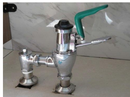
Figure 8b. Dual flush toilettes
