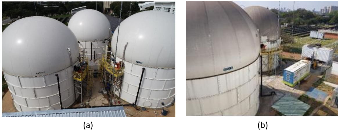
Figure 1. Images of the bioenergy and fertilizer production plant installed at IEE-USP (a) CSTR biodigesters and (b) Electric power generation units.
