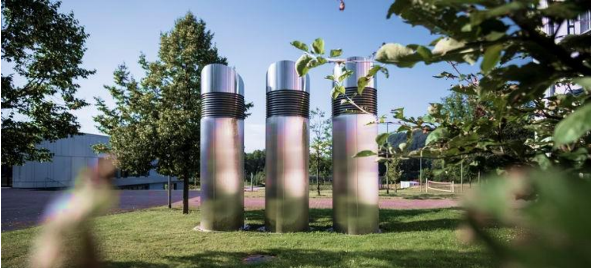
Figure 4. Air-intake for the central building
