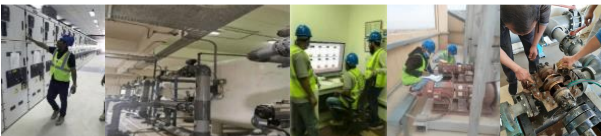
Figure 14. Monitoring distribution water Piping network in Qassim Campus.
