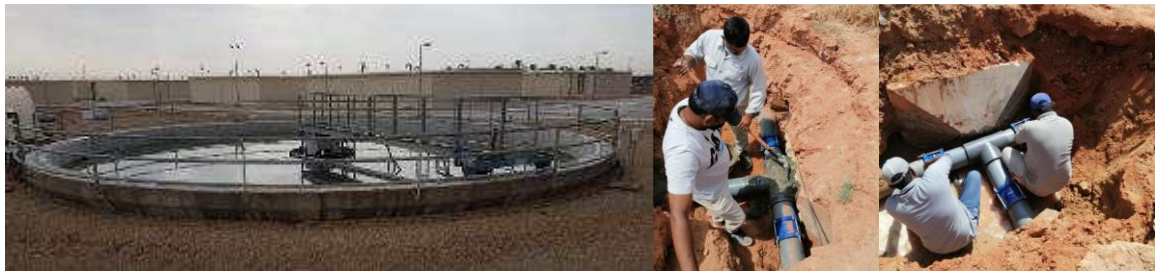
Figure 9. Final settling basins.
