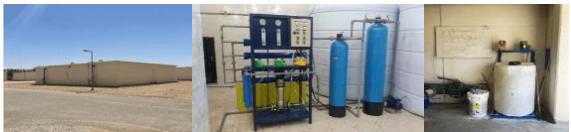
Figure 11. Irrigation water tanks and Sterilization unit.
