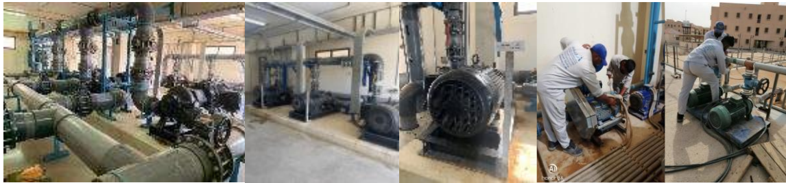
Figure 12. Pumps for pumping treated water.
