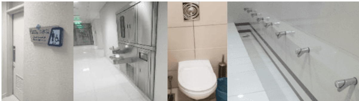
Figure 18. Some water efficient appliances in Qassim University.
