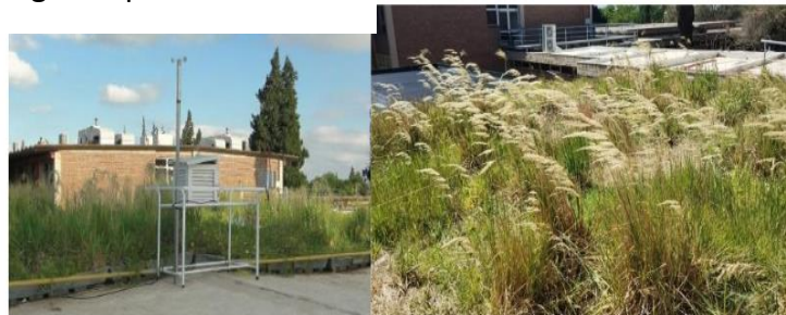
Figure 7: Location of the green roof in the workshop classrooms of the University's Faculty of Architecture. Images of the green roof with the weather station and the vegetation in its current state (age of the green roof: 5 years). Own source: UCC press archive
