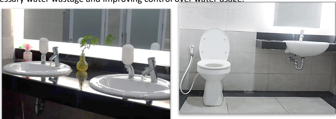
Figure 3. Water-saving equipment installed at UIN Raden Intan Lampung
