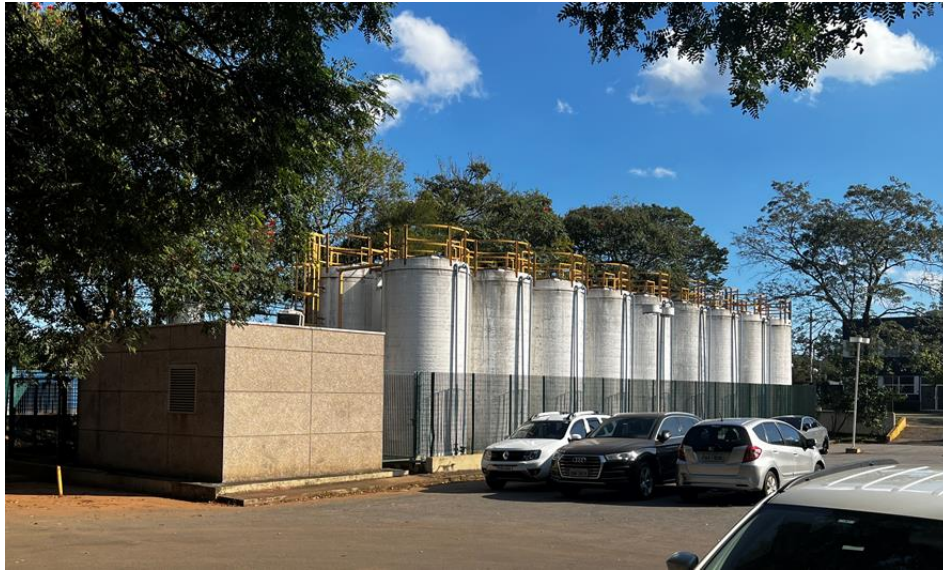
Figure 2. Sewage Treatment Plant (STP) of Centro Universitário Senac – Campus Santo Amaro. Source: own authorship.
