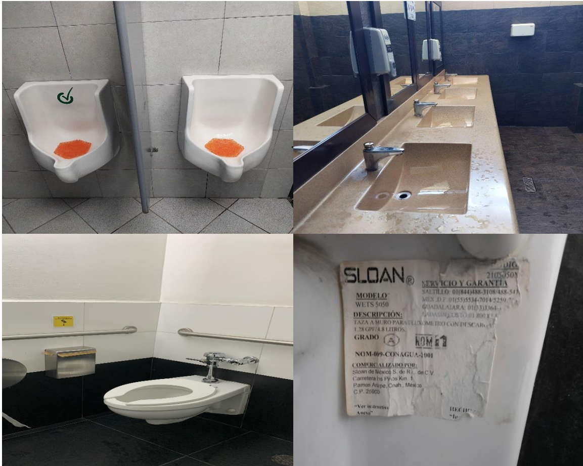
Figure 4. Water-efficient appliances at CETYS University (evidence)
