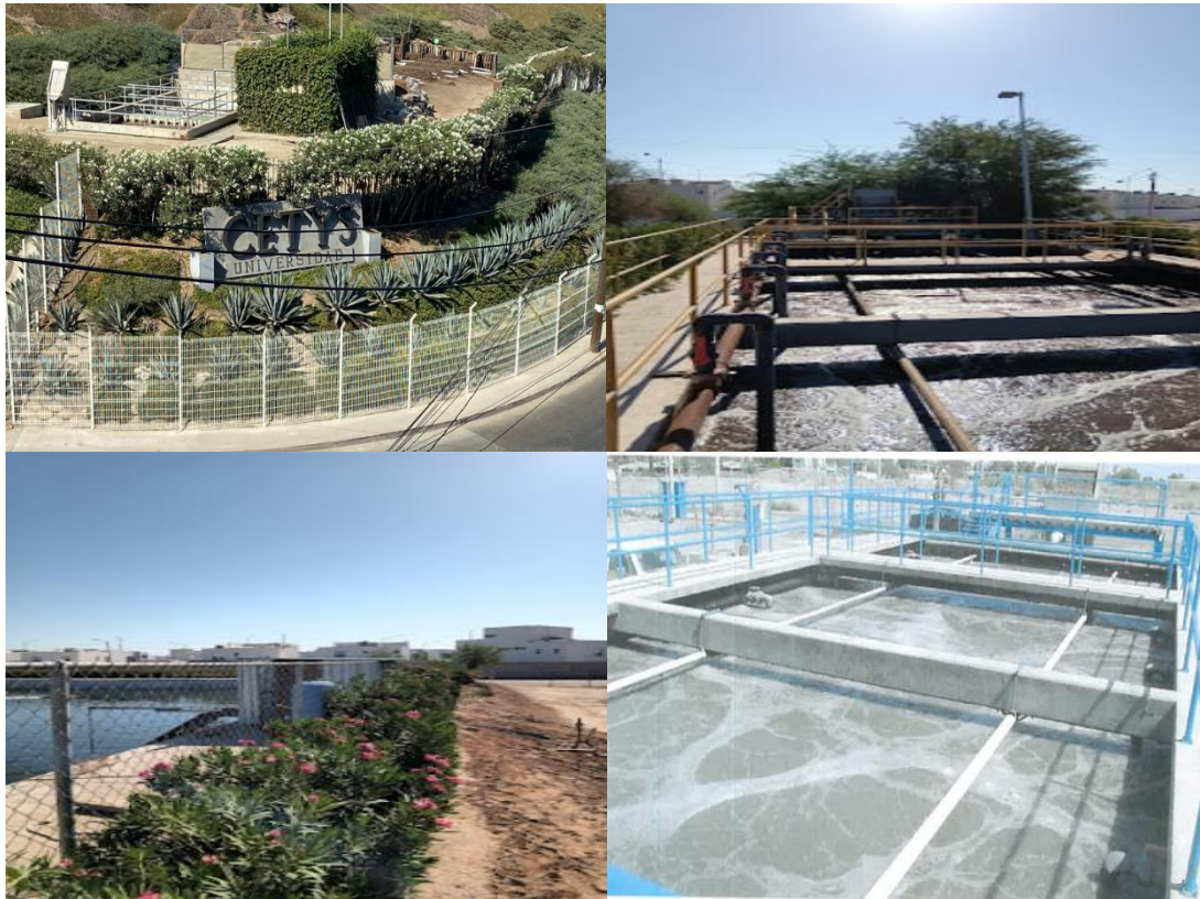
Figure 3. CETYS Tijuana and Mexicali campus wastewater treatment plants
