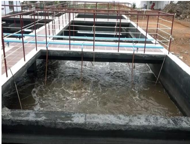
Figure 7. Aeration Basin of Sewage Treatment Plant
