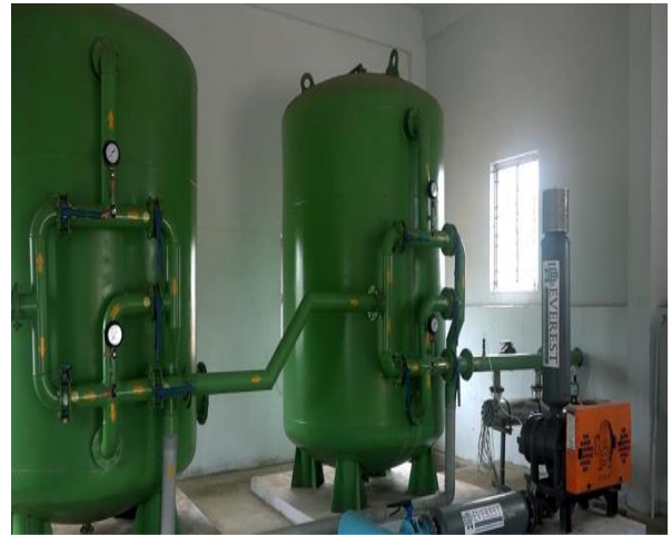
Figure 8. Tertiary treatment of sewage water using rapid sand filter, activated charcoal, UV and Chlorine disinfection
