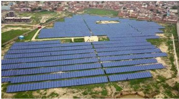
Figure 1. 3.3 MWp Grid Integrated Solar Farm at AMU
