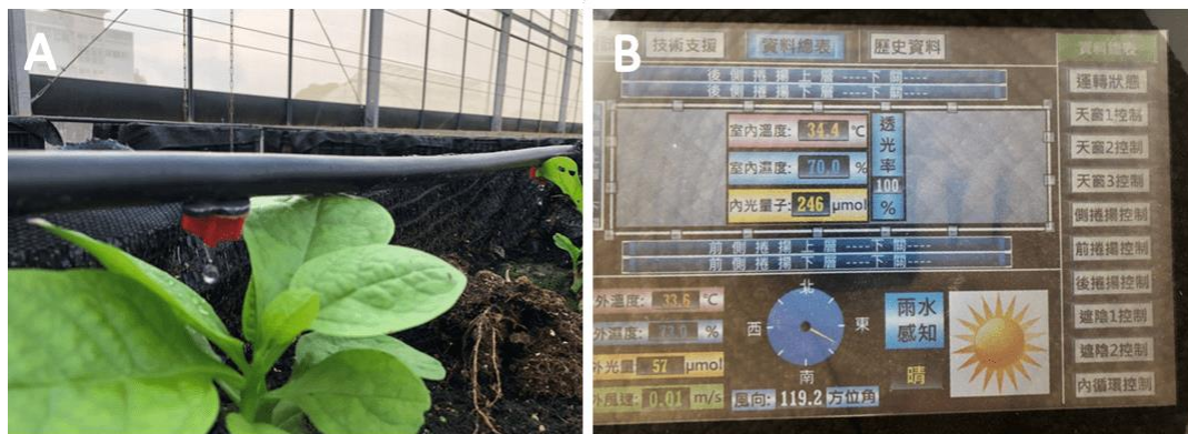
Figure 3. Smart irrigation system. A. Drip irrigation facility. B. A real-time monitoring system
