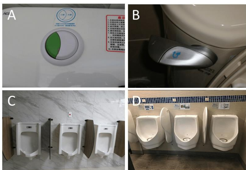
Figure 2. Water-saving appliances. A&B. Dual flush toilet, C. Urinals with sensors, D. Nano-coating non-flushing urinal.
