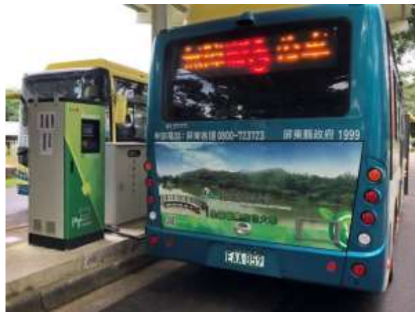
Figure 4. Electric Bus charging at the station
