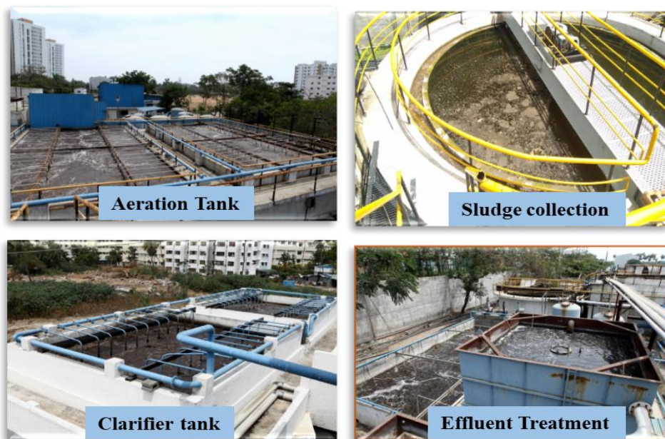
Figure 2. STP Treatment plant
