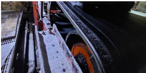
Gambar 6. Transfer conveyor (Sumber: PT Pupuk Indonesia Logistik)
