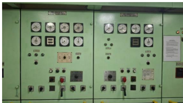
Gambar 2. Main switch board KM MPM (Sumber: PT Pupuk Indonesia Logistik)
