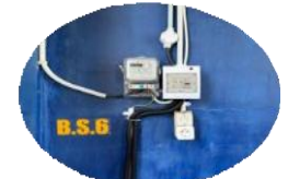
Panel listrik (449 unit)
