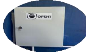
Operation system hydromechanical internet based (OPSHI) (665 unit)
