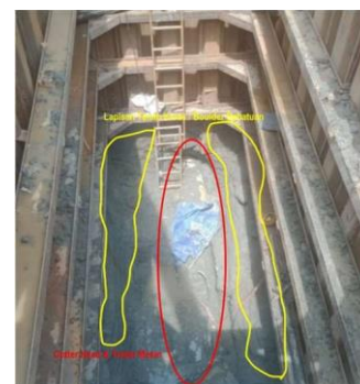
Gambar 12. Rescue pit MH 3001A
