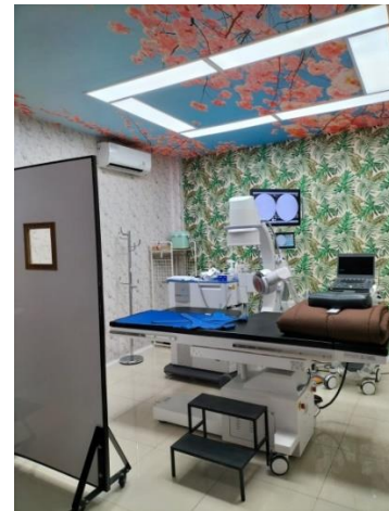
Fig. 5: ESWL room at XYZ Hospital
