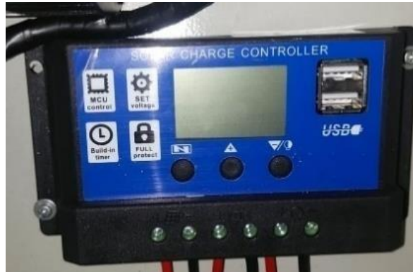
Gambar 5. Solar Charge Control
