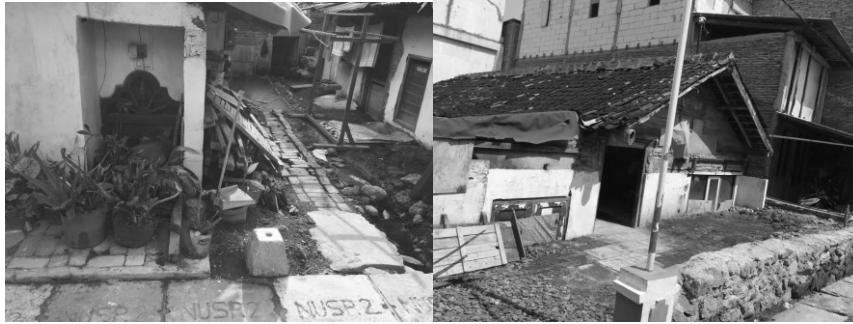
Figure 3. Sinking Houses in Kaligawe Slum Area (Source: Survey Documentation, 2018)
