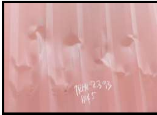
Figure 2 Damage Straighten THRU6892393
